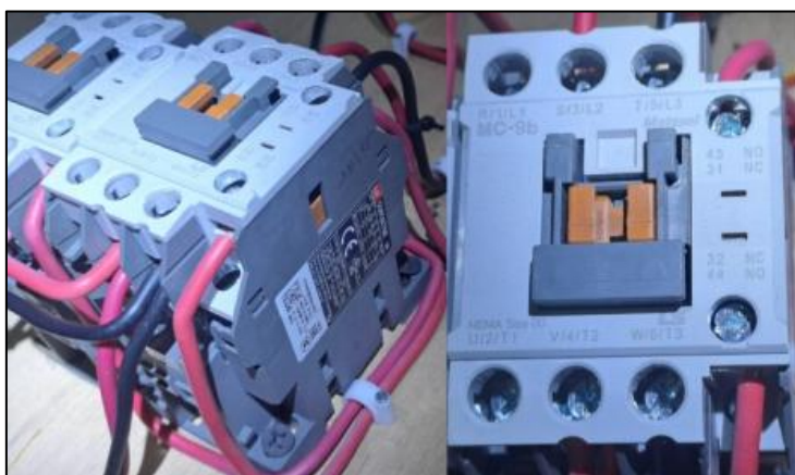
Fig. 6: The contactors used
